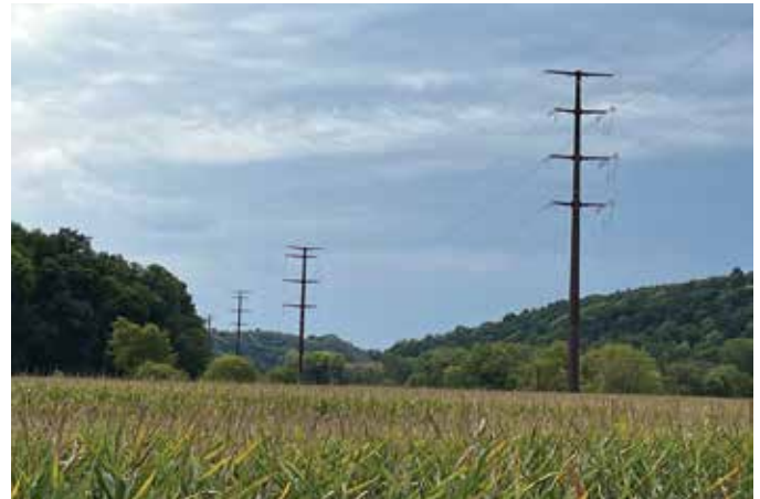
Pictured above: A portion of the Cardinal-Hickory Creek transmission line in Grant County, WI.
